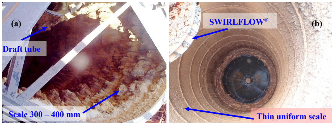
Figure 9. Photos of scale formed in a) draft tube and b) SWIRLFLOW® after the precipitation tanks taken offline for service.
